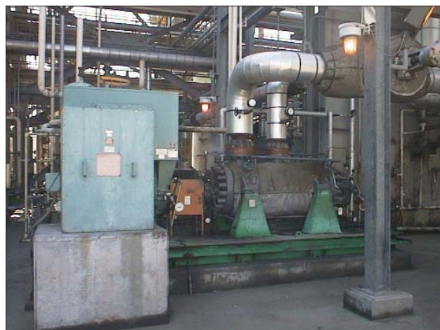
Figure 1. Rerated pump with increased performance installed and operating at the customer's site.
