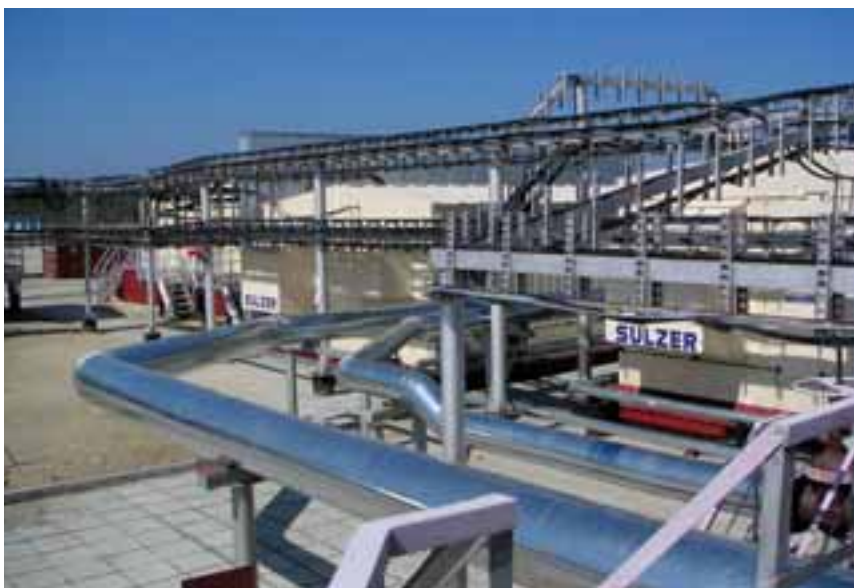
Pumping station in Western Siberia: three MPPs operating in parallel.
