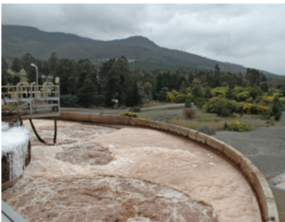
HST 6000 feeds 9 units of OKIs with air in the activated sludge tank.
